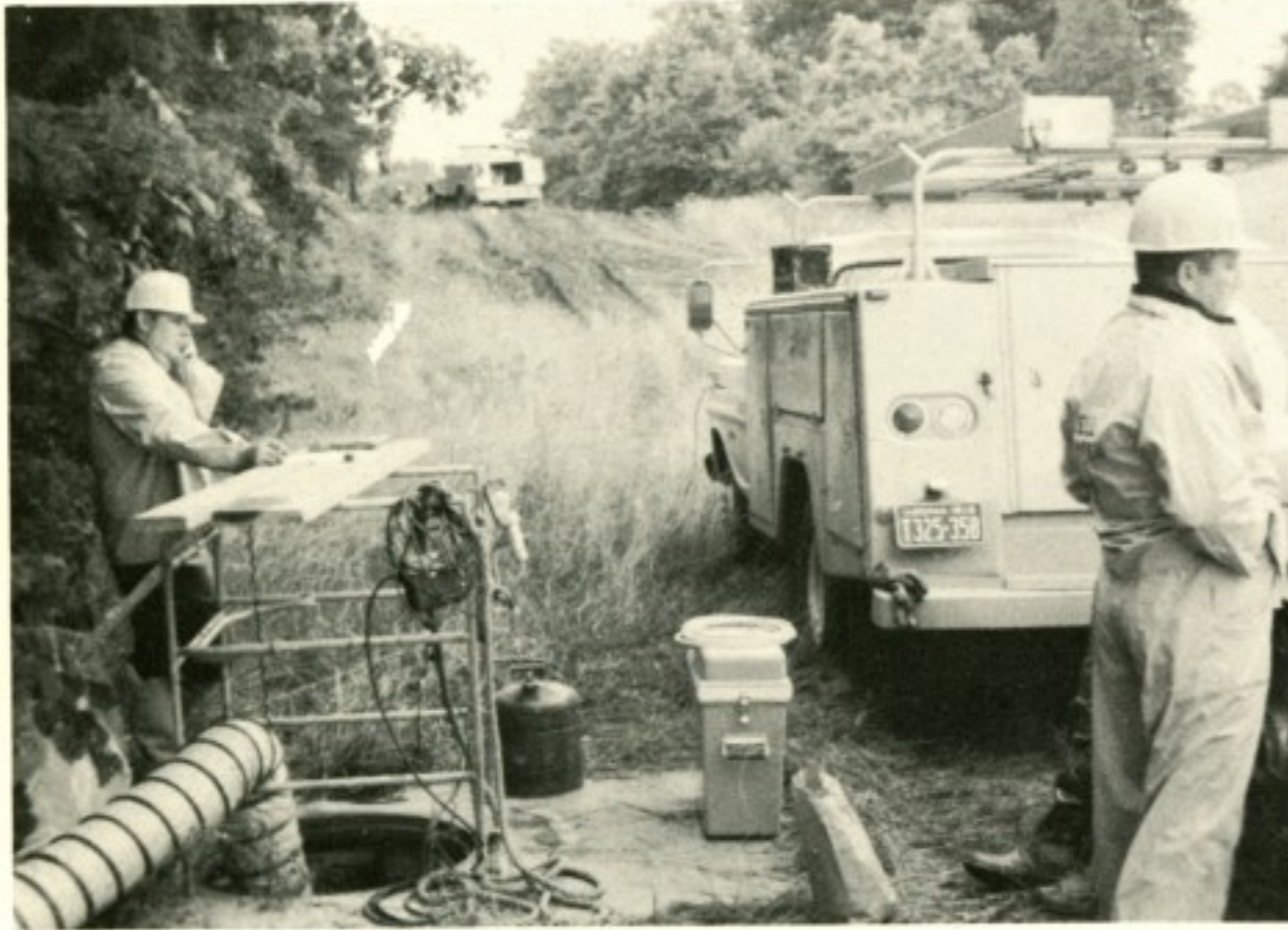
Flood and damage caused by Hurricane Agnes in 1972 near Dulles Airport. Long Lines forces from the Richmond District are shown in the restoration process.
