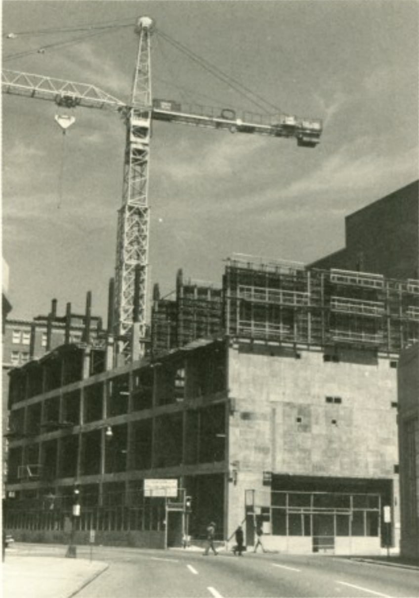
Bute Street building under construction after earlier problem with cave-in of foundation.
