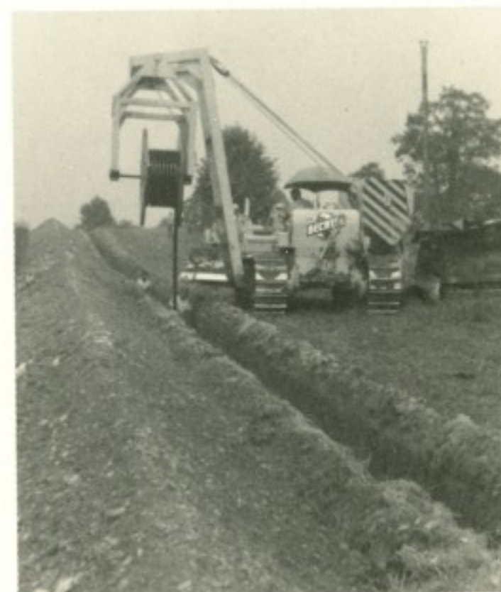
L4 cable being laid on the Moseley-Stanfield section of the Boston-Miami route.
