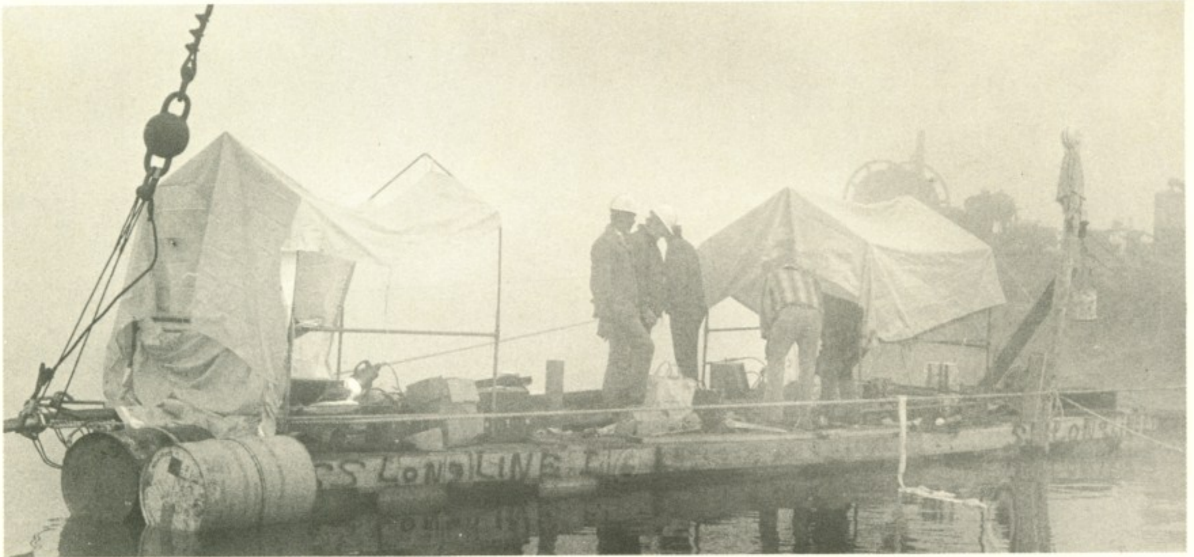
This barge was constructed in the fog by Long Lines forces during cable break of the Rappahanock which was caused by a commercial barge mashing the cable. The homemade rig was christened "SS Long Lines #2"
