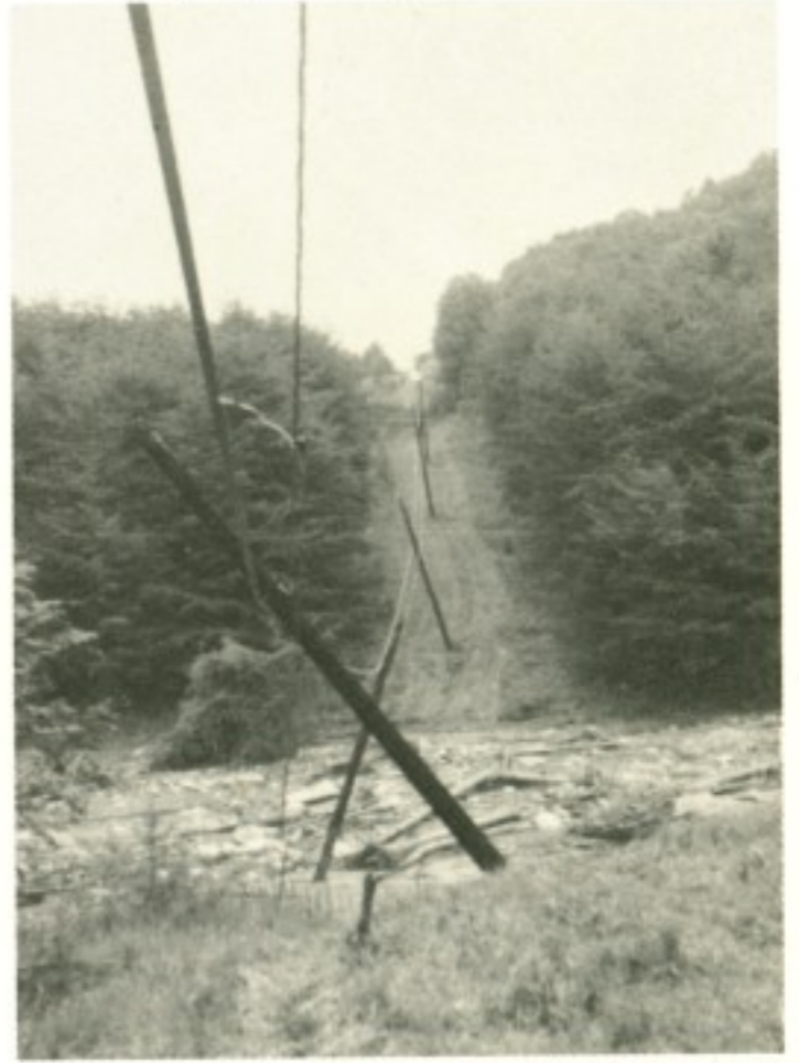
These pictures show damage done by Hurricane Camille in Nelson County. The flood and mud slides resulted in damage to 5 sections of the Upper Strasburg-Lynchburg Cable.
