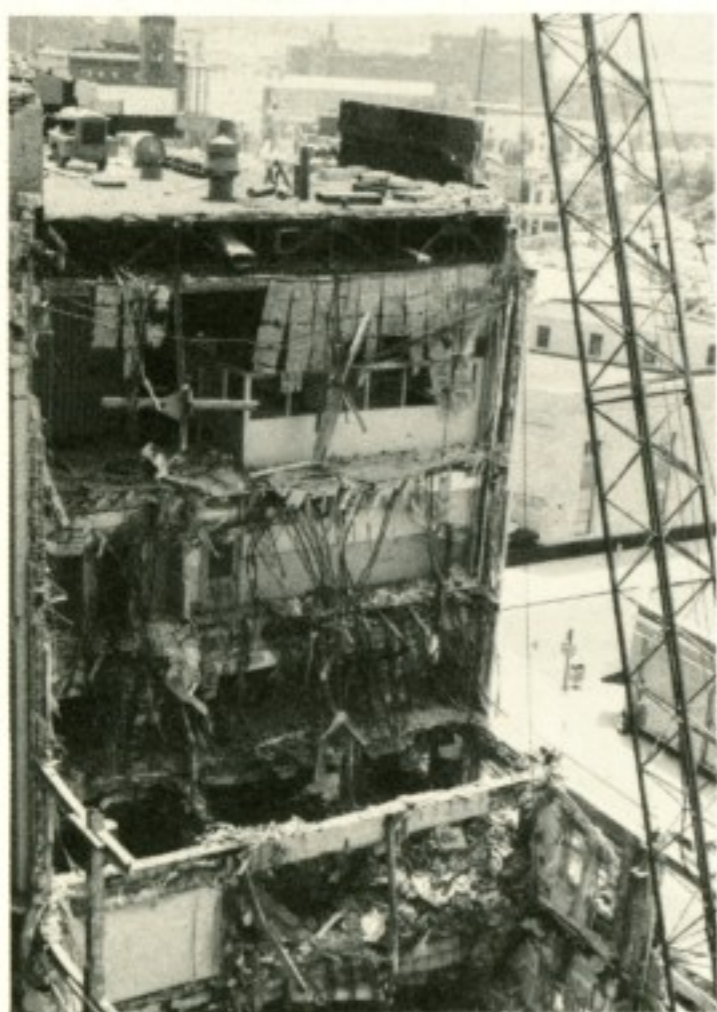
1969 demolition of the old Virginia National Bank in Norfolk, making way for addition to the Bute Street office.
